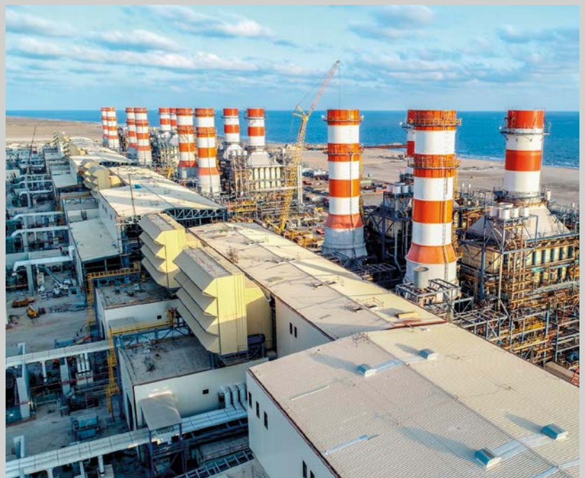
Combined Cycle Power Plant (CCPP) in Beni Suf, Egypt
